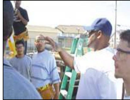
Lester Royal, gesturing with his arm, addresses members of a Summit Academy Opportunities Industrialization Center construction class as they rebuild a shed at a work site in Minneapolis. Royal, a licensed journeyman from Los Angeles, is one of the instructors at the facility.
